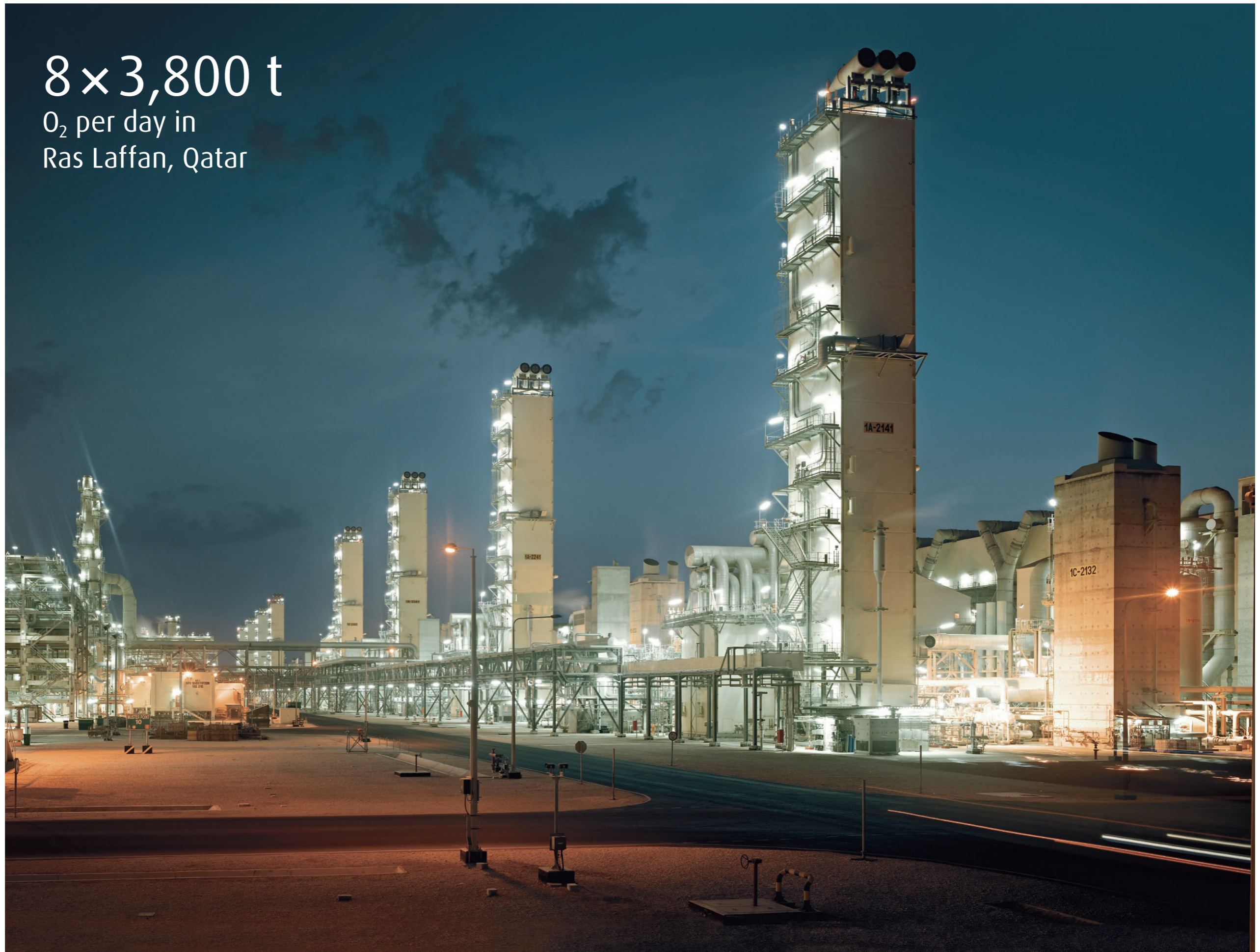
Air separation units at the Pearl GTL complex in Ras Laffan, Qatar.
